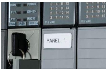
Control Panel Labels
