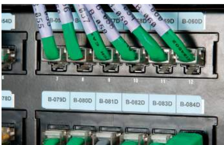
Patch Panel Labels
