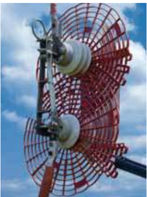
BISG-24 energized install
