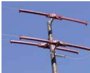
2 Pieces: MVLC-38 on busbar with BCIC
