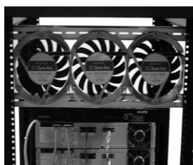
Fig.7 Photograph Showing Three Developed Products Mounted in a 19-inch Rack (EIA standard)
