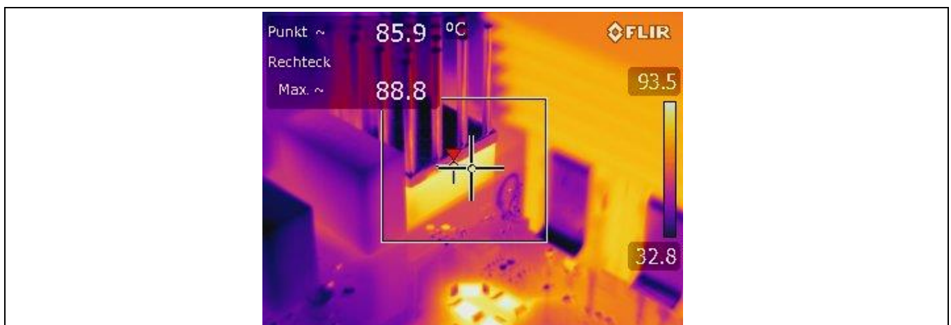
Figure 32 Thermal image of the input rectifier
