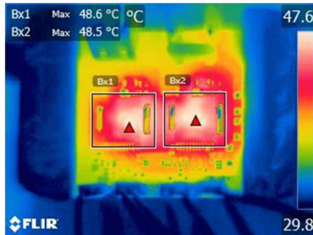
Figure 21 – Thermal Scan at 15 W Inverter Output in External-Supply Operation.
