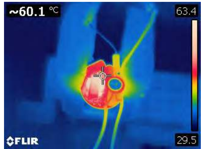
Figure 39 – 300 VAC, 48 V LED Load. Spot 1: EMI Inductor (L1): 60.1 °C.
