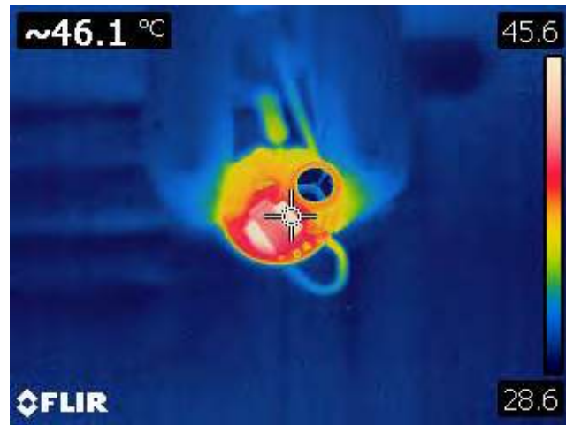
Figure 41 – 115 VAC, 67 V LED Load. Spot 1: Inductor (T1): 74.2 °C.
