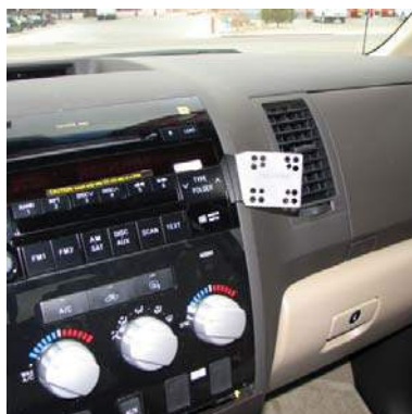
Final Installation Picture
