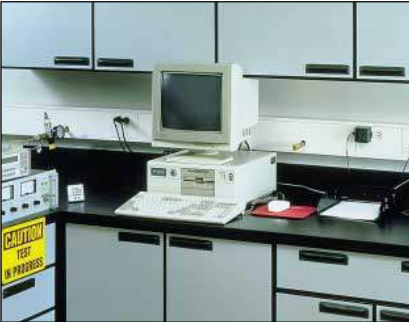
With a large capacity and multichannel capability, PAN-WAY Type T Surface Raceway can integrate both power and communication cabling systems while maintaining a neat and professional appearance throughout a testing lab.
