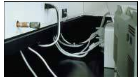
To further organize cables, use Type T Raceway in conjunction with PANDUCT® Type G Wiring Duct to route and conceal device cable slack.
