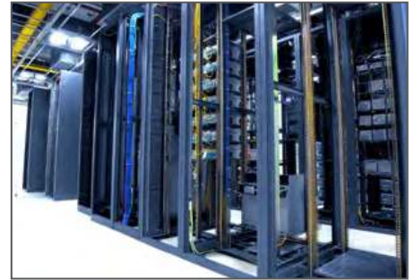
Servers, routers, switches, data centers and more
