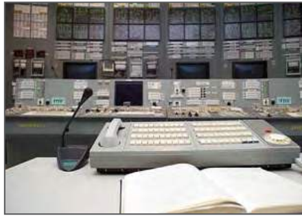
Programmable logic control systems
