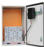
RPST with 100Ah of battery
