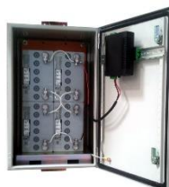
RPST with 200Ah of battery
