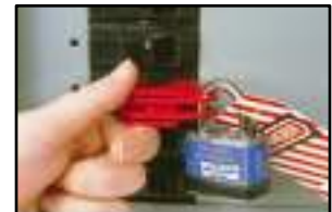
Verify that the lockout device secures the disconnect in a safe or off position.
