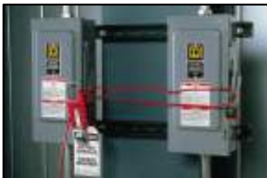
Lockout Single or Multiple Disconnects
