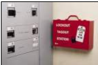
Mount close to power and distribution panels
