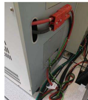
UPS Power Consumption Monitoring
