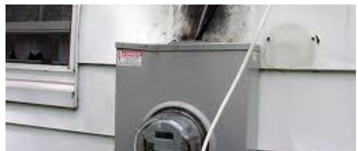
Service entrance destroyed by a surge
