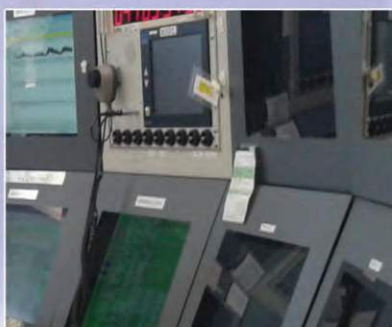
Stations Control Technology
