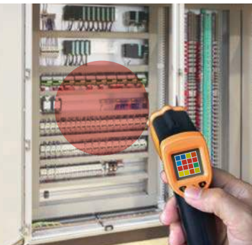
Transformers & distribution boards
