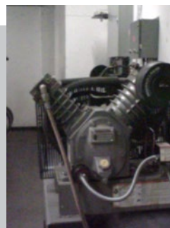
Air Compressor – Full Visible
