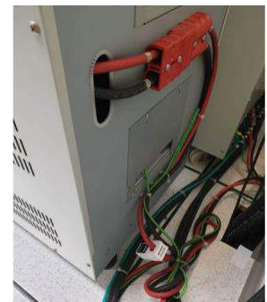
UPS Power Consumption Monitoring
