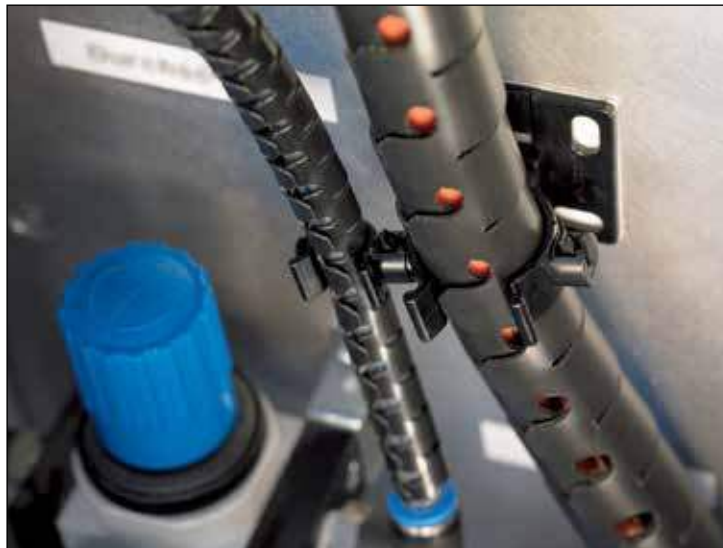
For example: The protection and affixing of cables in a wiring cabinet with Helawrap sleeving.
