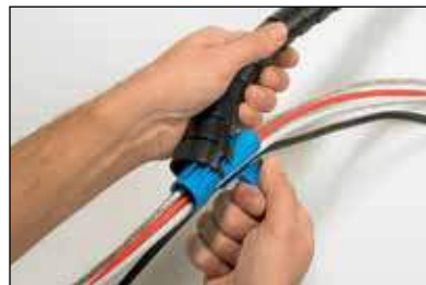
Place the applicator tool in one end of the Helawrap cable sleeving.
