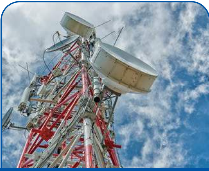
Telecom -Data Infrastructure
