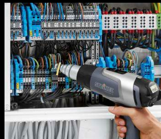
Shrinking cable sleeves in distribution cabinet
