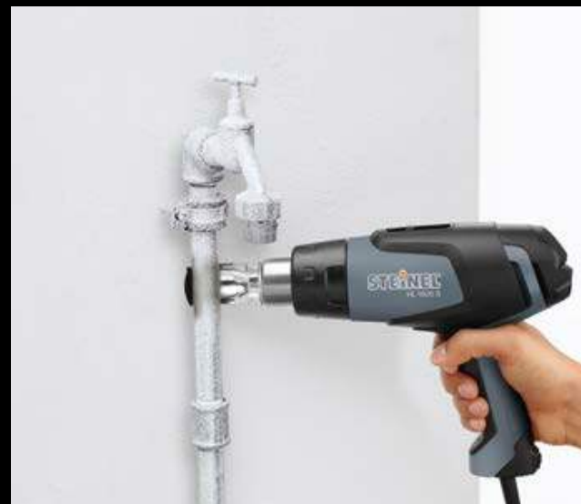
Thawing frozen pipes.
