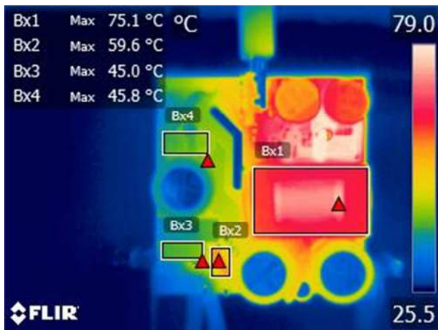
Figure 35 – Top Thermal Image, T_{AMB} = 26.9\text{ }^{\circ}\text{C} . Bx1: Transformer, T_1 = 75.1\text{ }^{\circ}\text{C} . Bx2: Thermistor, RT_1 = 59.6\text{ }^{\circ}\text{C} . Bx3: CMC 1, L_1 = 45.0\text{ }^{\circ}\text{C} . Bx4: CMC 2, L_2 = 45.8\text{ }^{\circ}\text{C} .
