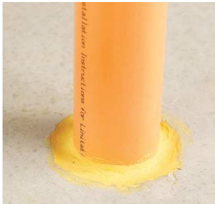
Firestop metal or CPVC fire sprinkler lines: 3M™ Fire Barrier Sealant IC 15WB+ ( pg 32 )
