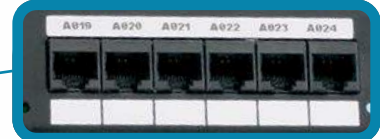
Patch Panel / Face Plate Labels
