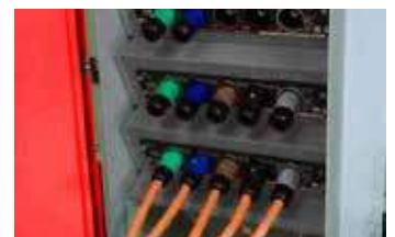
Emergency power systems
