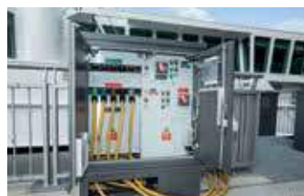
Dock power distribution systems
