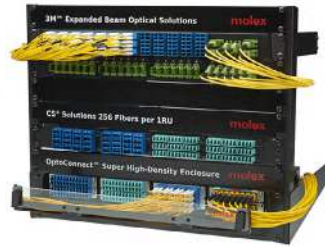
Data Center Rack
