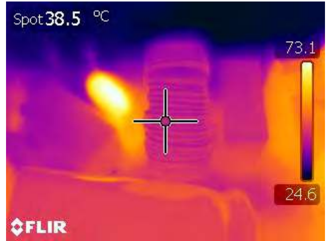
Figure 70 – Common Mode Choke (L1), 230 VAC Input, 100% Load, Room Temperature.
