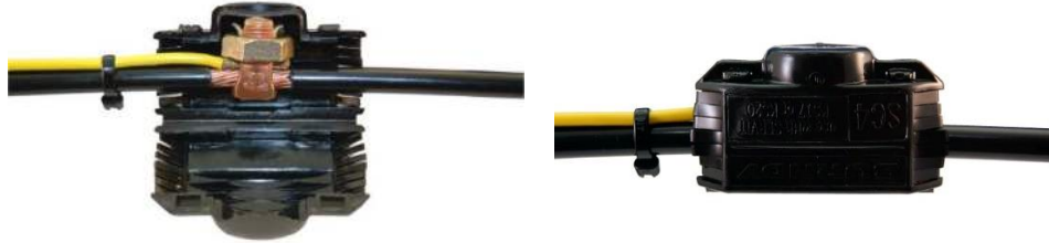
Figure 1: Sensor leads are secured with cable ties near the termination point
