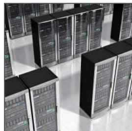
Data Center Servers
