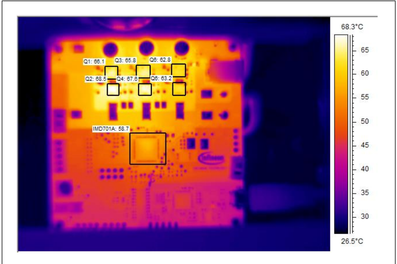
Figure 64 Thermal measurement summary at 18 V input and 300 W load
