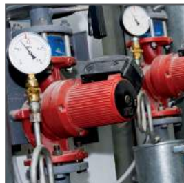
Sensors, valves and control cabinets
