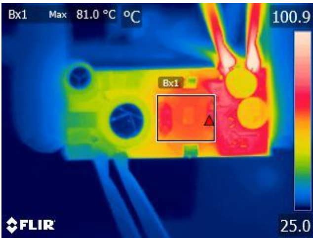
Figure 42 – Ambient = 25 °C. Transformer, T2 = 81 °C.
