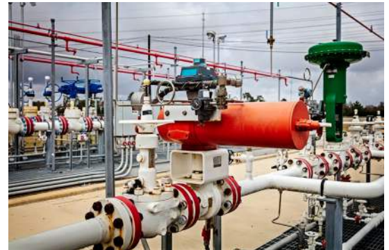
Figure 1. Industrial Valve Application
