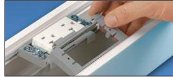
T130DBD installed in Type T raceway
