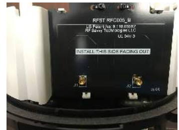
Fig 1.0 AMC-RFCRFS005B-A RF Coupler Installed in kV2C Meter
