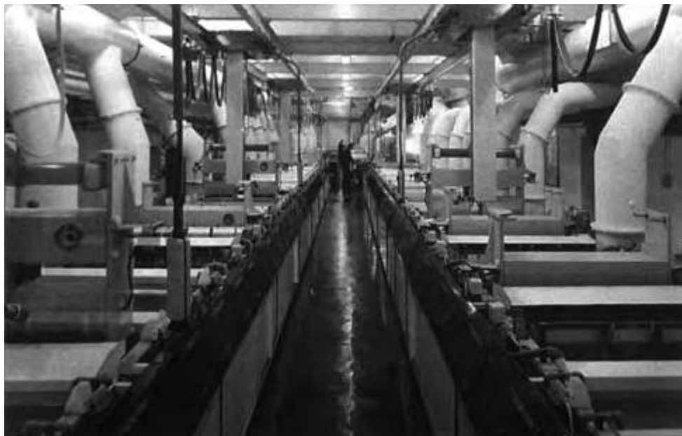
Tyco Electronics' industrial electroplating facilities is one of the most advanced in the world.
