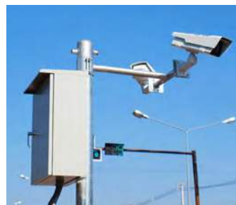
Traffic Control & Surveillance
