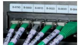
Patch panel labels
