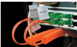
Fiber optic cable markers
