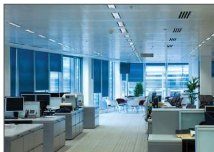
LED office lighting
