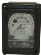
1. Old Meter in Panel
