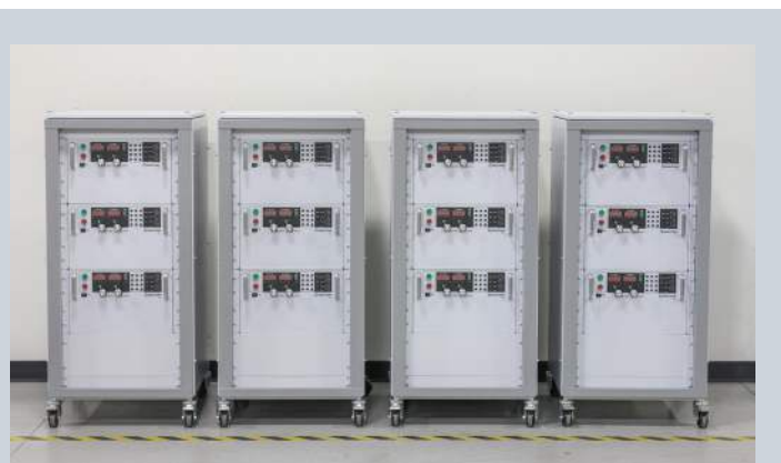
Qty (12) 30 kW TS Series with water cooling (+WC) packaged in Qty (4) CAB2
