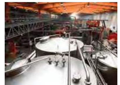
Millions of dollars are lost every year in the food and beverage industry from production line damage and lost productivity when hoses and wires are damaged by rodents.
