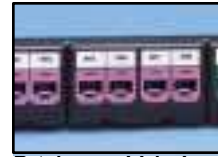
Patch panel labels
