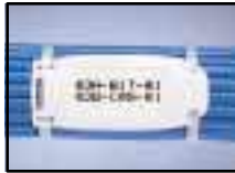
Cable bundle labels
